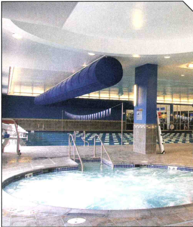
In an effort to reach sustainability goals, the HUMC Fitness and Wellness Center installed a pool dehumidification system using glycol, reducing refrigerant use by 80%.
